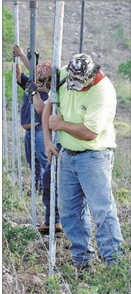
Workers pound fence posts in January 2010 as part of the Pelekane Bay Watershed Restoration Project. - WHT File Photo
